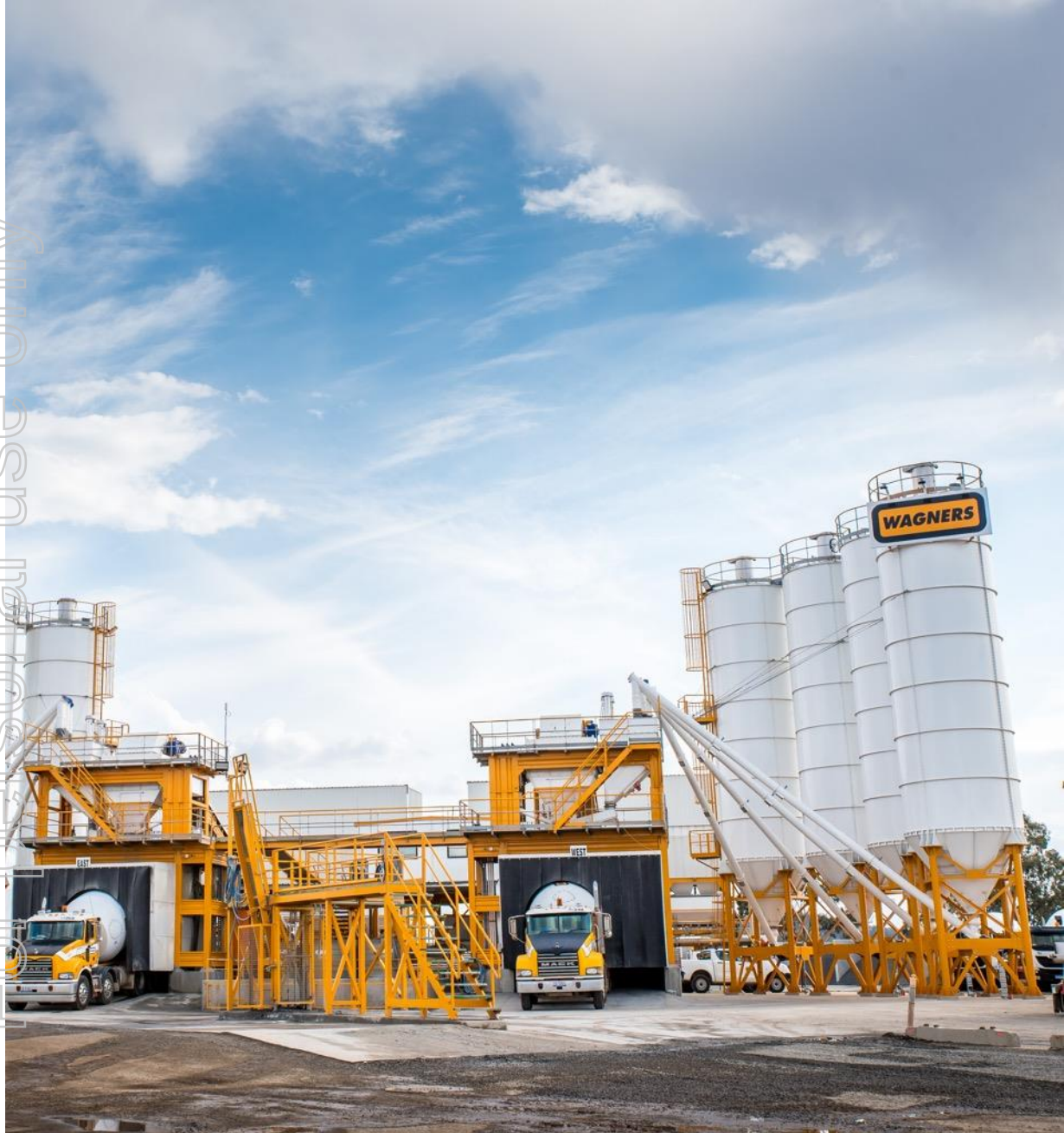
Batch Plant and Agitators at Toowoomba Batch Plant, QLD
